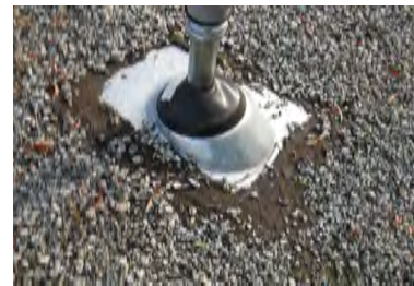
Typical Deficiency - Through roof penetrations do not appear to have proper roof jack. Recommend installing proper roof jack and storm collar.
