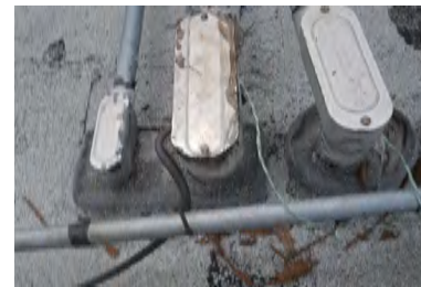
Typical Deficiency - LB electrical penetrations have not been flashed properly. Recommend installing galvanized pitch pocket with cover.
