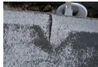
Typical Deficiency - BUR at gravel stop edge metal has split at joints. Recommend removing loose material to expose adequate tie-in of existing striping plies, prime and re-flash per industry standards.
