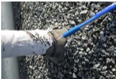
Typical Deficiency - Detailing at through roof penetrations show signs of cracking and delamination. Recommend touch up of mastic at penetrations and application of acrylic or silicone coating to preserve and maintain repair.
