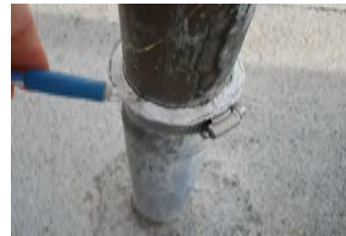
Typical Deficiency - Sealant at lead pipe jacks has begun to pull away from through roof penetration. Recommend replacing sealant as needed, installing stainless steel band clamps, and storm collar.
