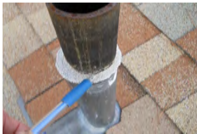
Typical Deficiency - Pipe jack sealant has begun to pull away from through roof pipe penetration. Recommend application of flexible flashing self-adhered tape and sealant, and install storm collar.
