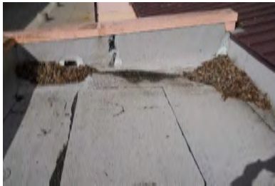
Typical Deficiency - Debris have accumulated at field of roof. Recommend clearing debris from all gutters, drains, waterways, and field of roof to promote positive drainage. Through wall scuppers should have debris screens. Recommend installation of gutter screens to promote positive drainage.
