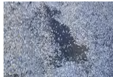
Typical Deficiency - Areas of displaced gravel. Recommend re-distributing and adhering gravel over bare areas to protect underlying membrane from exposure to UV .
