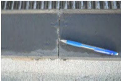
Typical Deficiency - Sealant at coping seams has begun to fail. Recommend removal and replacement of sealant as needed.
