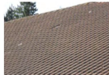
Typical Deficiency - Missing concrete S tile. Recommend replacement of all missing and or damaged tiles.
