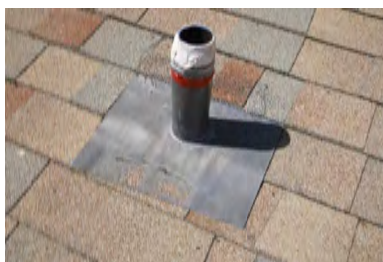
Typical Deficiency - Through roof penetration does not appear to have proper roof jack. Recommend installing proper roof jack and storm collar.
