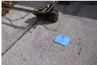
Typical Deficiency - Mineral surfaced cap sheet has blistered. Recommend relief cutting blister, imbed in layer of modified mastic, and apply target sheet of mineral surfaced cap sheet in cold applied adhesive.
