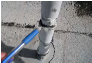
Typical Deficiency - Through roof penetration has not been properly sealed. Recommend re-sealing and installing storm collar.
