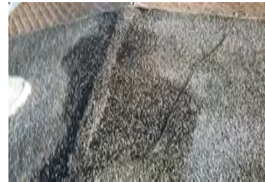
Typical Deficiency - Areas of displaced gravel. Recommend re-distributing and adhering gravel over bare areas to protect underlying membrane from exposure to UV .
