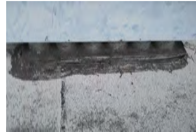
Typical Deficiency - Pitch pockets have dried up and sealant has pulled away from galvanized sheet metal flashing. Recommend removal and replacement of sealants.
