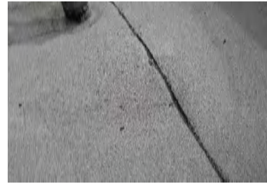
Typical Deficiency - Mineral surfaced cap sheet has blistered. Recommend relief cutting blister, imbed in layer of modified mastic, and apply target sheet of mineral surfaced cap sheet in cold applied adhesive.
