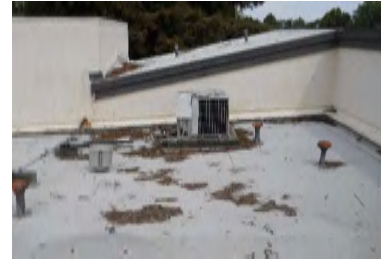
Typical Deficiency - Debris have accumulated on roofs. Recommend clearing debris from all gutters, drains, waterways, and field of roof to promote positive drainage.
