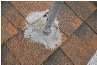
Typical Deficiency - Through roof penetrations do not appear to have proper roof jack. Recommend installing proper roof jack and storm collar.
