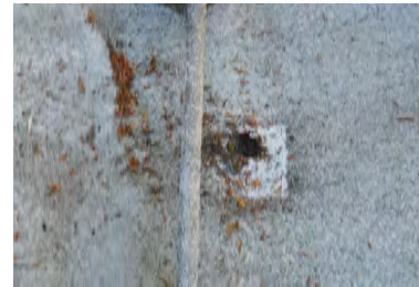
Typical Deficiency - Coating has begun to delaminate from foam roofing. Recommend touch up as needed.
