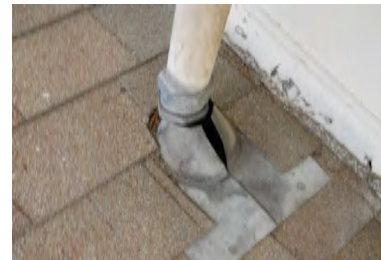
Typical Deficiency - Pipe jack is open. Recommend removal and replacement and installation of storm collar.
