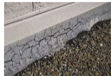
Typical Deficiency - Base flashings show signs of deterioration and cracking. Recommend application of silicone or acrylic coating to maximize usable life of existing built-up roof system.
