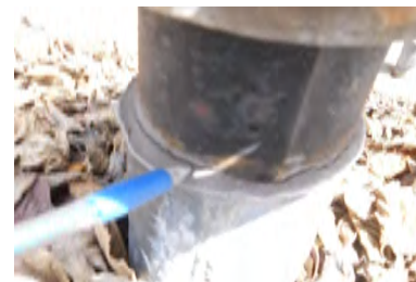
Typical Deficiency - Lead pipe jacks are missing band clamps and sealant. Recommend installing stainless steel band clamps, apply sealant, and install storm collar.
