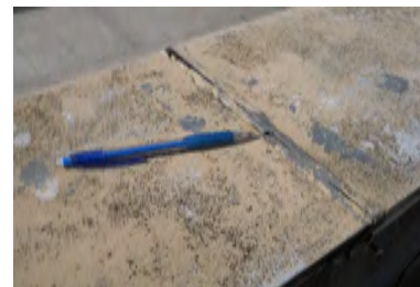
Typical Deficiency - Sealant at coping seams has begun to fail. Recommend removal and replacement of sealant as needed.
