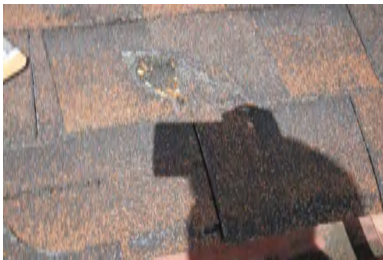
Typical Deficiency - Shingles are damaged. Recommend replacing as needed.
