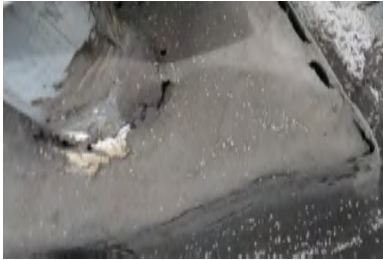
Typical Deficiency - Pitch pockets have dried up and sealant has pulled away from galvanized sheet metal flashing. Recommend removal and replacement of sealants.
