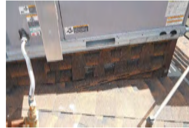
Typical Deficiency - Mechanical curbs have been improperly flashed. Recommend removal of shingles, install new sheet metal flashings properly tied into existing steep slope asphalt shingles.
