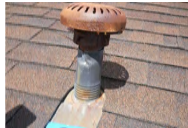
Typical Deficiency - Pipe jacks are missing band clamps and sealant. Recommend installing stainless steel band clamps, apply sealant, and install storm collar.
