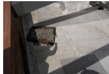
Typical Deficiency - Observed accumulation of debris at field of roof. Recommend clearing debris from all gutters, drains, waterways, and field of roof to promote positive drainage.
