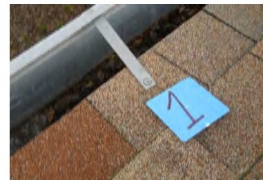
Typical Deficiency - Gutter brackets have been face fastened through asphalt shingle. Recommend removal and repositioning bracket. Repair asphalt shingles as needed.
