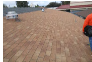
Typical Deficiency - Observed fastener penetrating through finished asphalt shingle roofing. Recommend removal and repair as needed.
