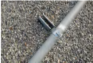
Typical Deficiency - Unistrut supports have been fastened directly through existing roof system. Recommend removal, repair of roof and refastening support to sleeper, floating block, etc..
