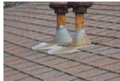
Typical Deficiency - Pipe jacks are missing band clamps and sealant. Recommend installing stainless steel band clamps, sealant, and install storm collar.
