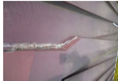
Typical Deficiency - Roof transition/ cricket has been temporarily sealed. Recommend removal of all temporary repairs and installation of as needed permanent repairs.
