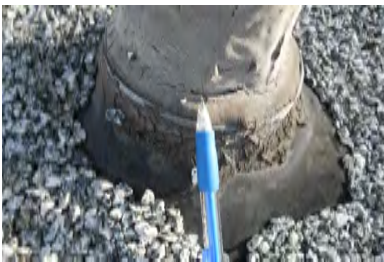
Typical Deficiency - Detailing at through roof penetrations show signs of cracking and delamination. Recommend touch up of mastic at penetrations and application of acrylic or silicone coating to preserve and maintain repair.
