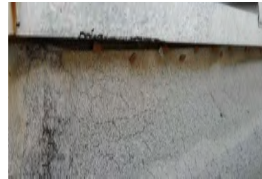
Typical Deficiency - Base flashing at mechanical curb has not been properly skirt flashed. Recommend installation of GSM skirt flashing.
