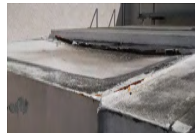
Typical Deficiency - Mechanical duct work damaged and deteriorated. Recommend replacement of damaged duct by licensed mechanical contractor and coating with acceptable silicone or acrylic coating.
