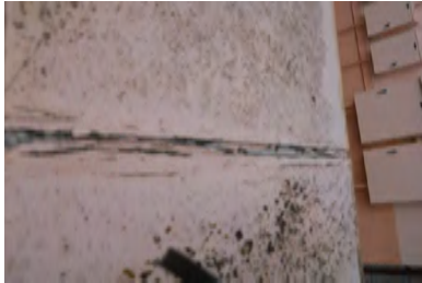
Typical Deficiency - Sealant at coping seams has begun to fail. Recommend removal and replacement of sealant as needed.
