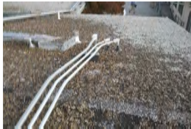
Typical Deficiency - Debris have accumulated at field of roof. Recommend clearing debris from all gutters, drains, waterways, and field of roof to promote positive drainage.
