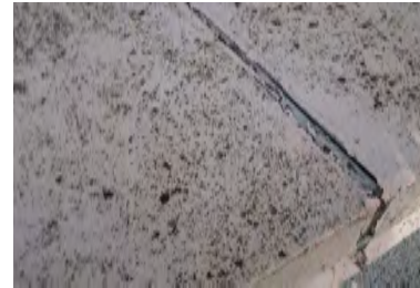
Typical Deficiency - Sealant at coping seams has begun to fail. Recommend removal and replacement of sealant as needed.
