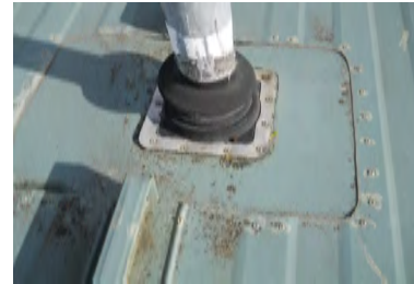
Typical Deficiency - Detailing at through roof penetrations show signs of cracking and delamination. Recommend touch up of sealants..
