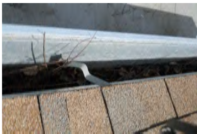
Typical Deficiency - Gutter straps need to be re-fastened.
