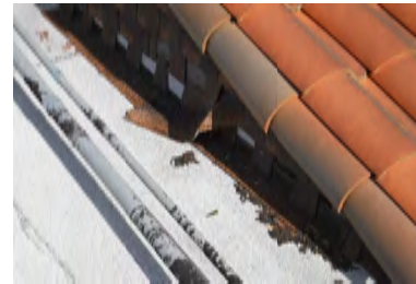
Typical Deficiency - Roof to wall transition has been improperly detailed. Recommend removing shingles and installing proper counterflashing assembly, roofing and wall finishes by others.
