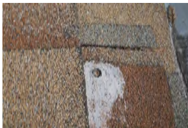
Typical Deficiency - Observed fastener penetrating through finished asphalt shingle roofing. Recommend removal and repair as needed.
